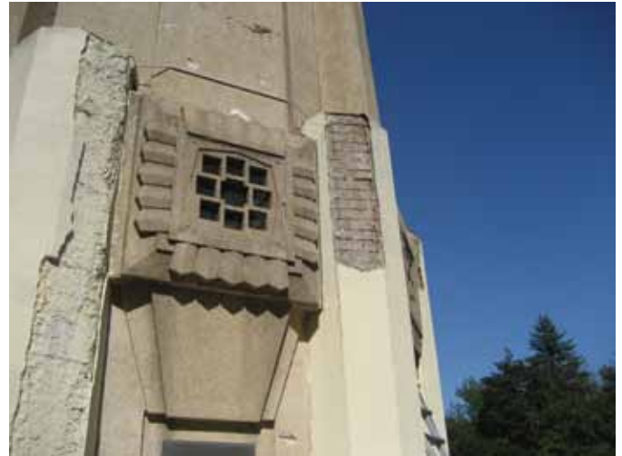
Field investigations at the Edison Memorial Tower revealed a range of deterioration caused by two factors: corrosion of the embedded reinforcing steel and cycles of freezing and thawing (Photo courtesy of Mills + Schnoering Architects, LLC)
