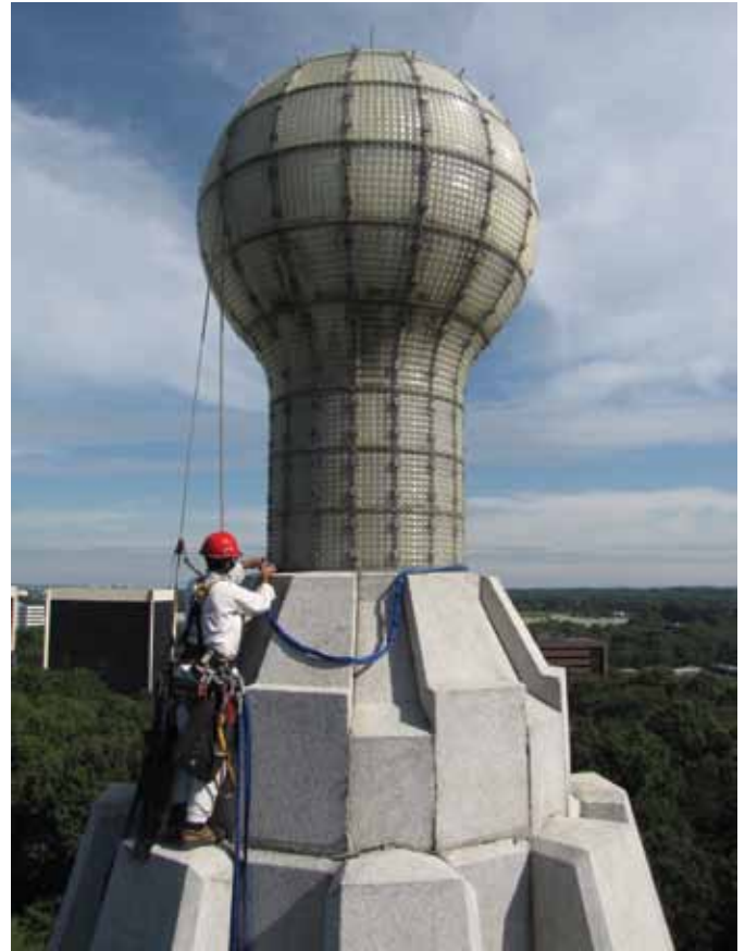
The concrete panels at the top of the Edison Tower are white with a cobalt blue color so they match the color of the sky. Closer inspection reveals the scale of the Pyrex replica of the light bulb. The light bulb will also be cleaned as part of the restoration process (Photo courtesy of Mills + Schnoering Architects, LLC)
