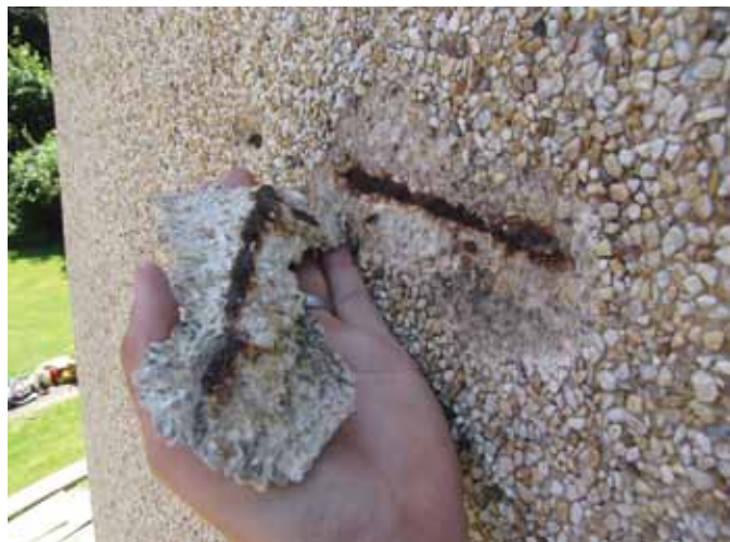
A corroded reinforcing bar behind the exposed aggregate concrete facing of the Edison Memorial Tower (Photo courtesy of Mills + Schnoering Architects, LLC)
