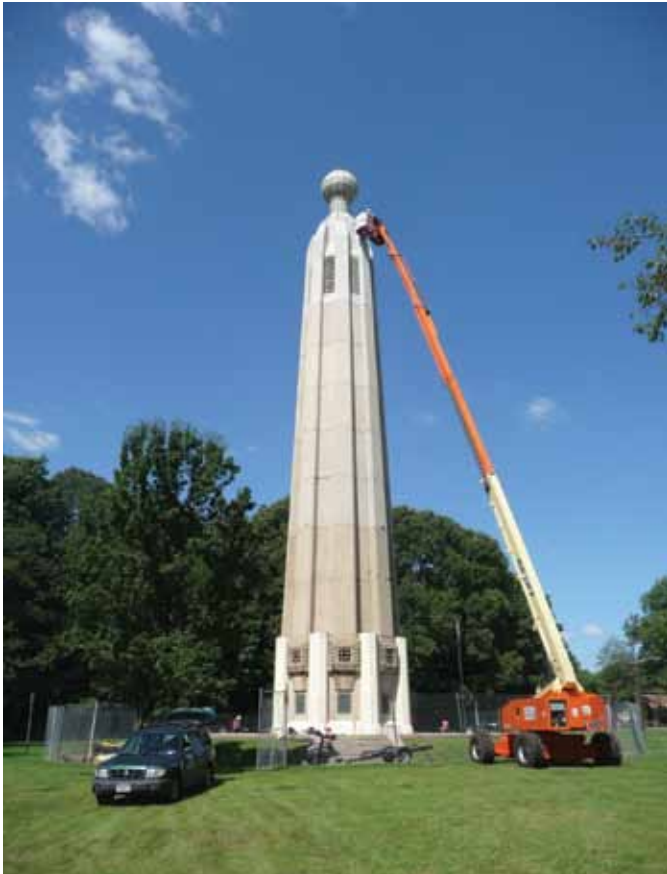
With its concrete heavily deteriorating, the state of New Jersey hired Mills + Schnoering Architects, LLC, to restore the Edison Tower. Field investigations in 2009 revealed that some panels, mostly the ones at the top, had to be completely replaced (Photo courtesy of Mills + Schnoering Architects, LLC)
