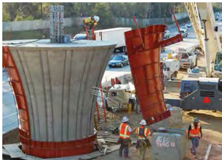
Workers strip the forms from one of three CIDH foundation piers. The pier flares provide a base for a 25 ft (7.6 m) tall basket feature
