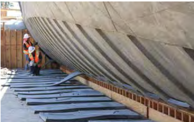
The bridge's ribbed design was created by fastening polymeric form liners onto curved forms. Here, workers pull the liners from the concrete
