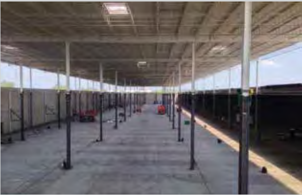
An example of capturing unused air space to enlarge an industrial facility (photo courtesy of John J. Bernauer, EZ Riser Roof Raising Services)
