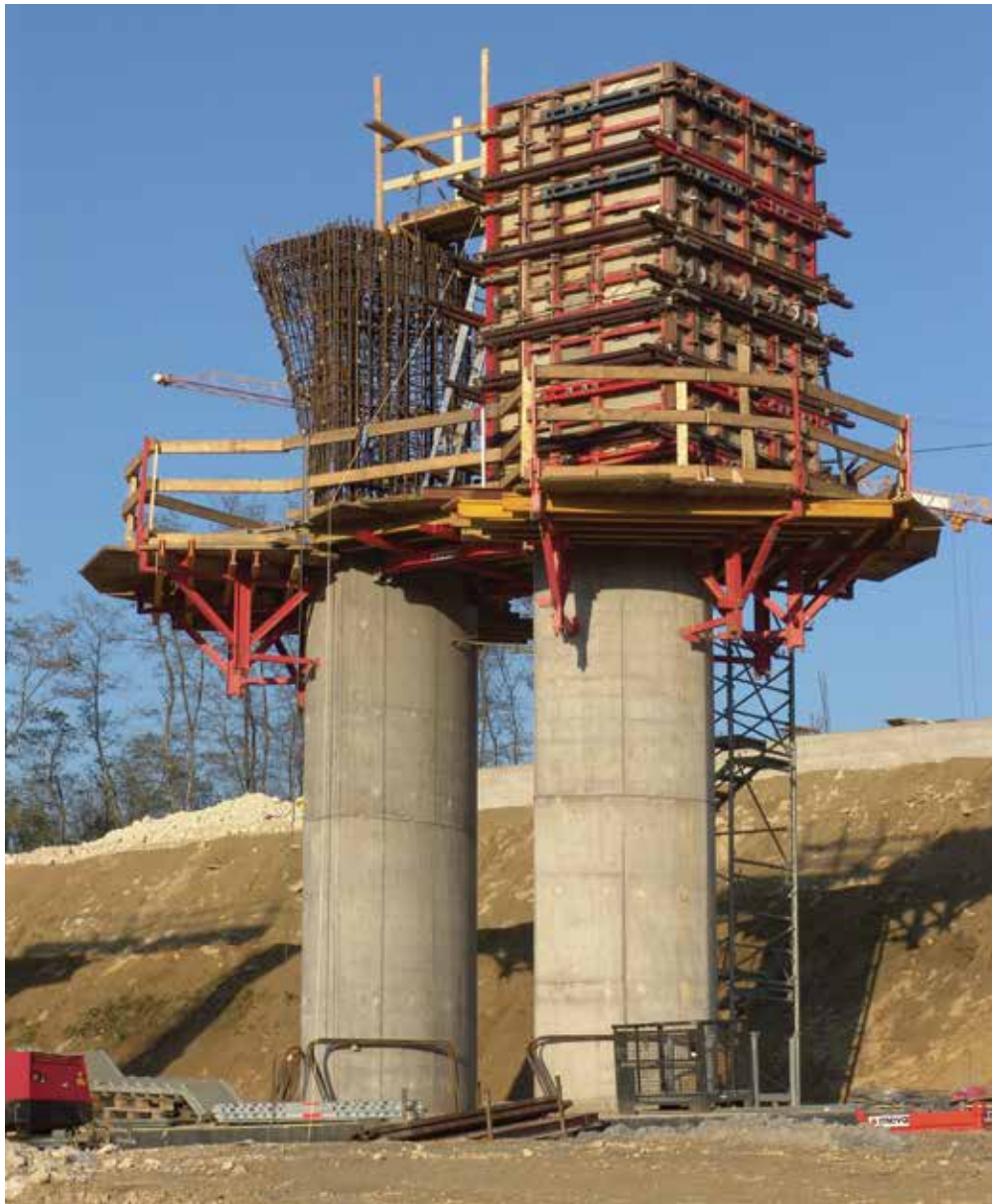
Fig. 15.15: External ties and full-span wales used to avoid internal ties (Photo courtesy MEVA Formwork Systems)
