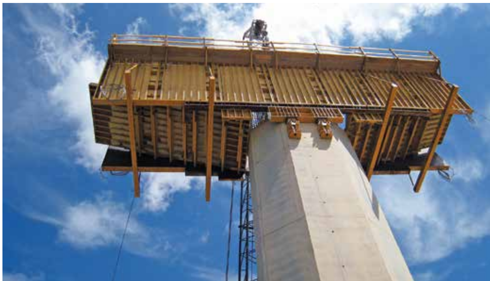
Fig. 15.16: Formwork for a hammerhead pier cap supported on brackets attached with through bolts (Photo courtesy EFCO Corp.)
